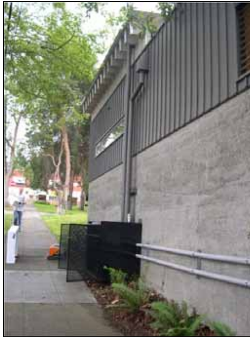
Figure 2-13 Photo Ross Park Shelterhouse Flow Monitoring Box, Located on the North Side of the Building
