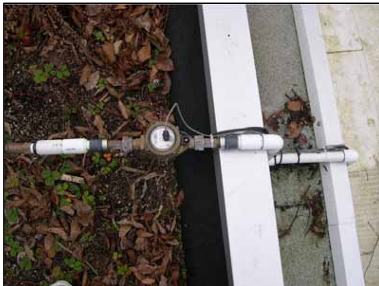
Figure 2-15 Multijet Meter Installed for Measurement of Irrigation Water Delivered to the Ross Park Shelterhouse green roof
