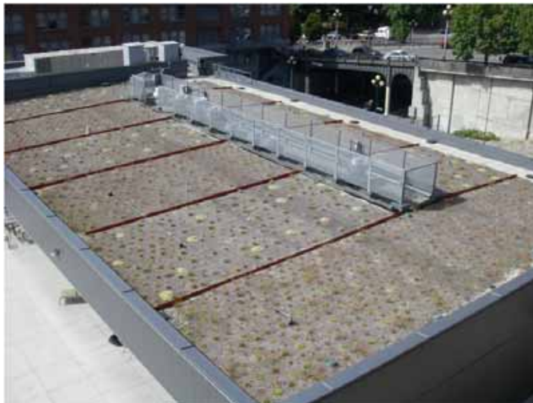
Figure 2-16 View of the Fire Station 10 Green Roof from the Emergency Operations Center Rooftop
