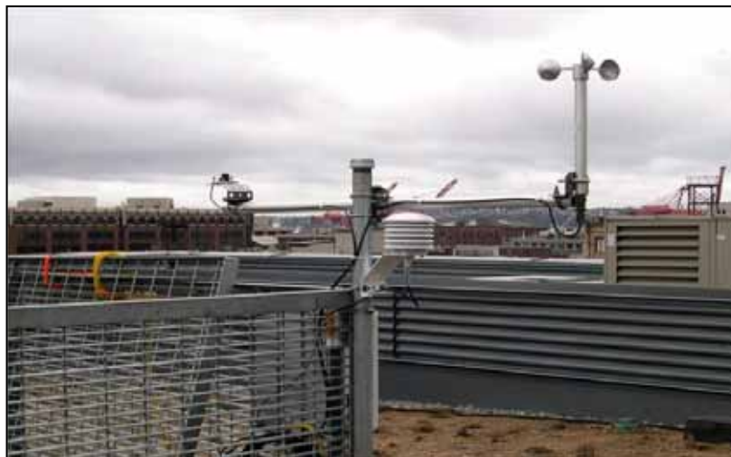
Figure 2-18 Meteorological Sensors (Weather Station) Installed on the FS10 Green Roof
