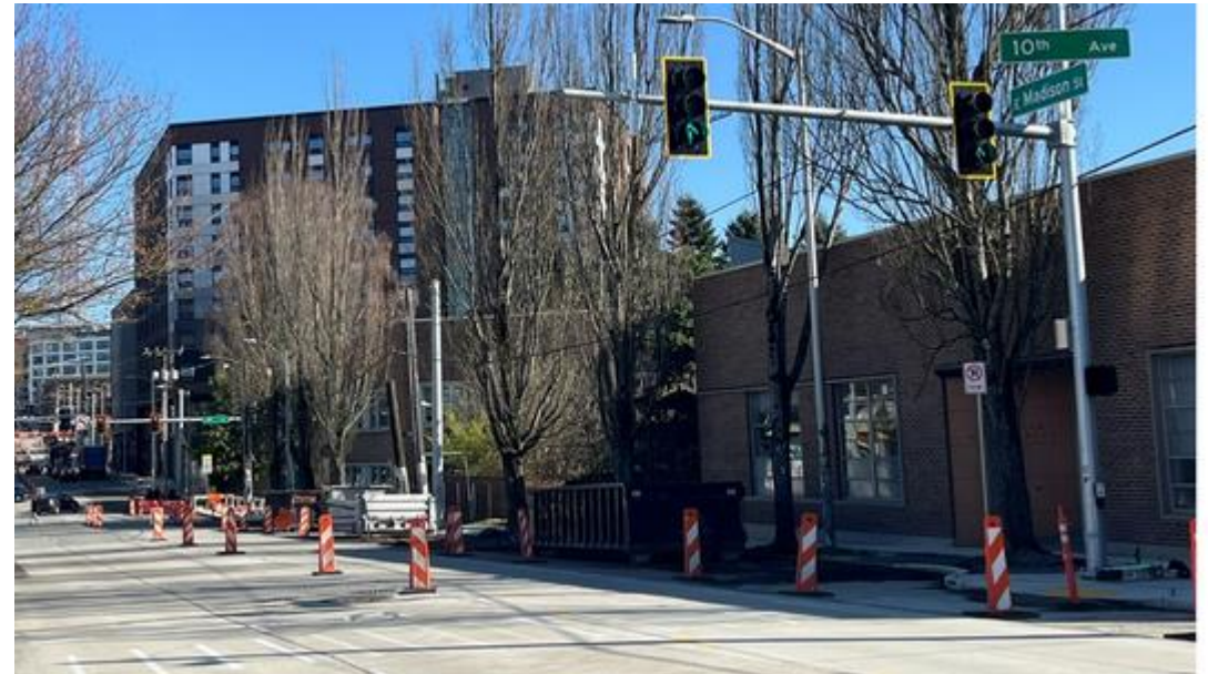
Bus shelter frame at 8th Avenue Bus Island and new signal at 10 th Ave and E Madison St as part of the Madison RapidRide G Line project.
