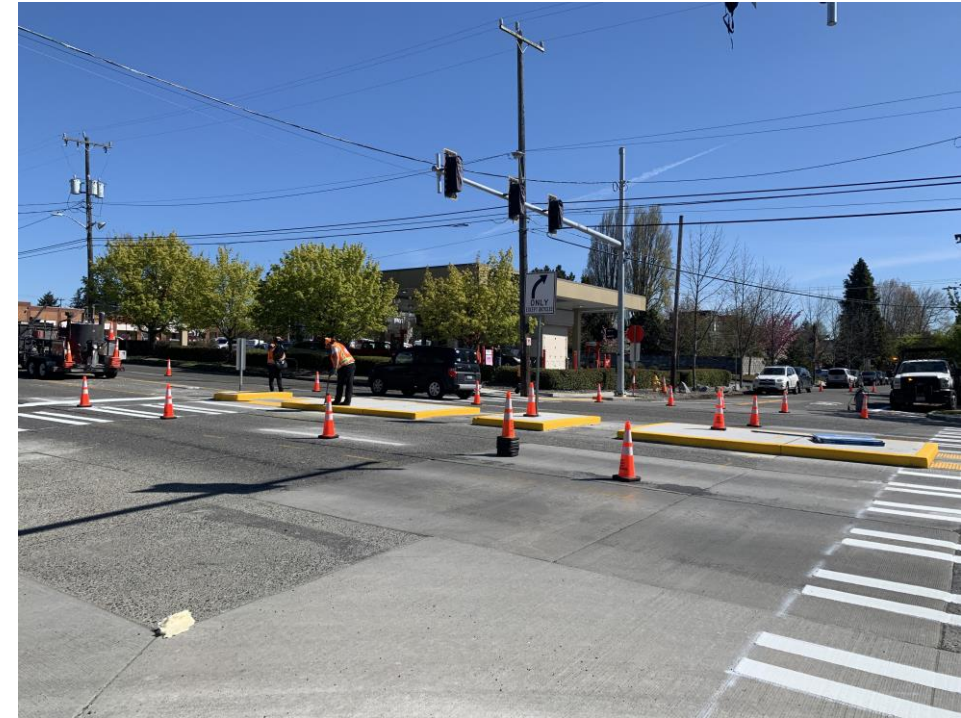
15 th Ave NW & NW 83 rd St Pedestrian Safety Enhancements NSF project under construction
